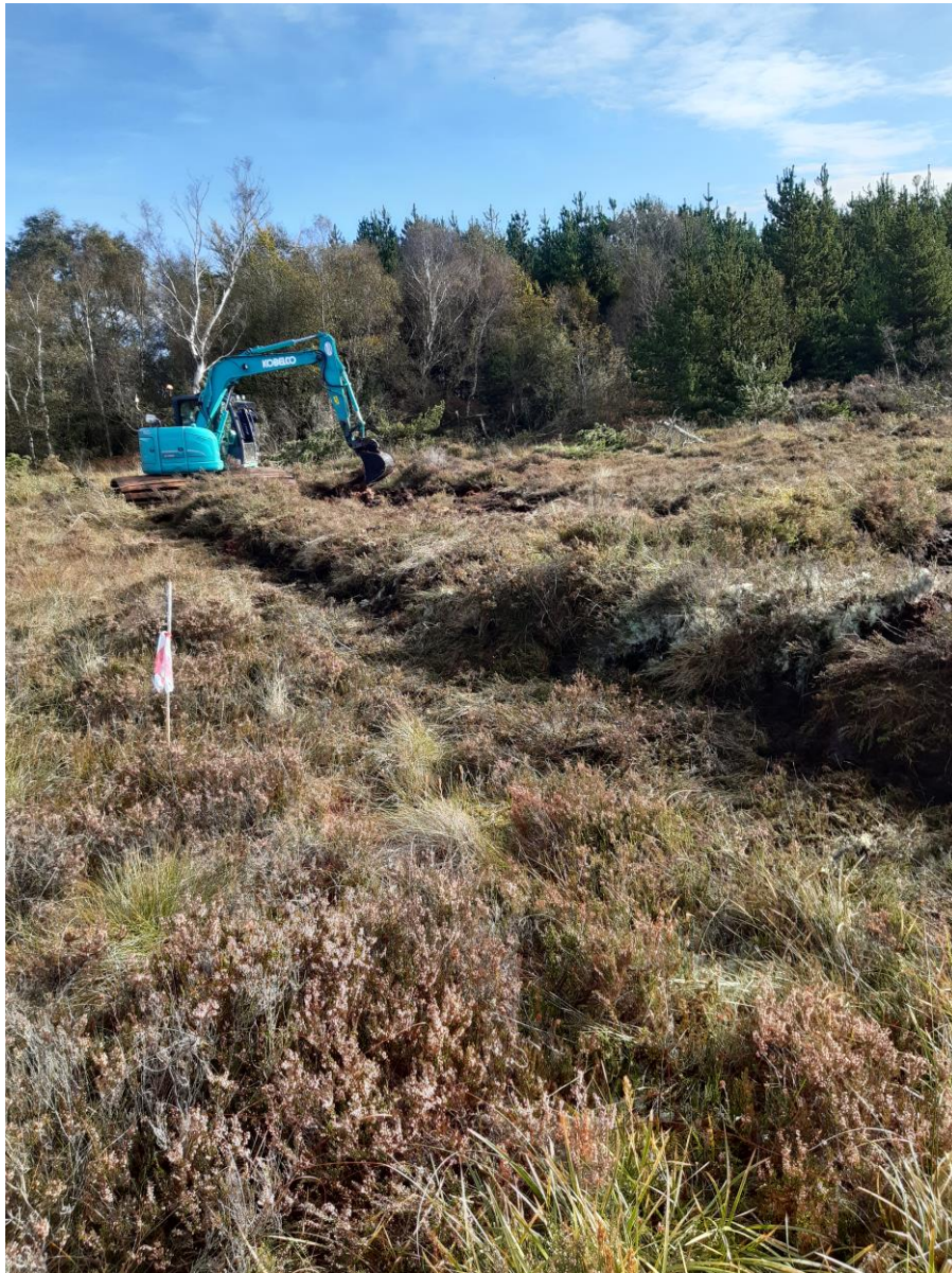
Figure 5.3 Example of setting out trench bunding on the cutover with bamboos and tape
