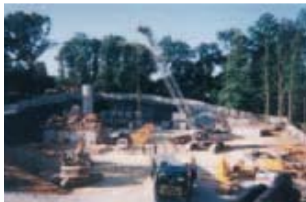
Located in an environmentally-sensitive zone, the site is particularly difficult to access.
