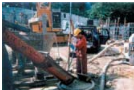
The upper part of the "Butard" shaft is excavated while being protected by a 1.02-m thick diaphragm wall.
