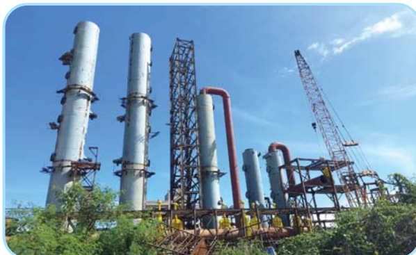
Coal Chemical Plant of Coke Oven Battery-5 - Scrubbing plant
