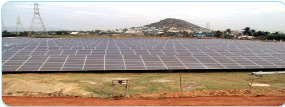
5MW ground mounted solar power PV (Photovoltaic) plant at Kanithi Road, RINL/VSP
