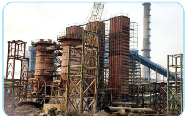
Coal Chemical Plant of Coke Oven Battery-5 - Primary Gas Cooler Electrostatic Tar Precipitator Area
