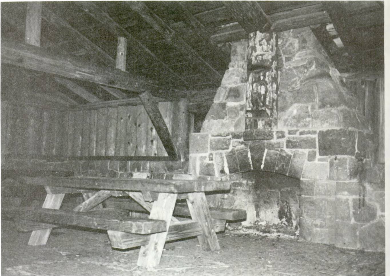
Figure 144--Back walls filled with upright logs, Bear Springs Picnic Shelter, Mount Hood National Forest, OR. (Photo by Dennis Egner, 1982)
