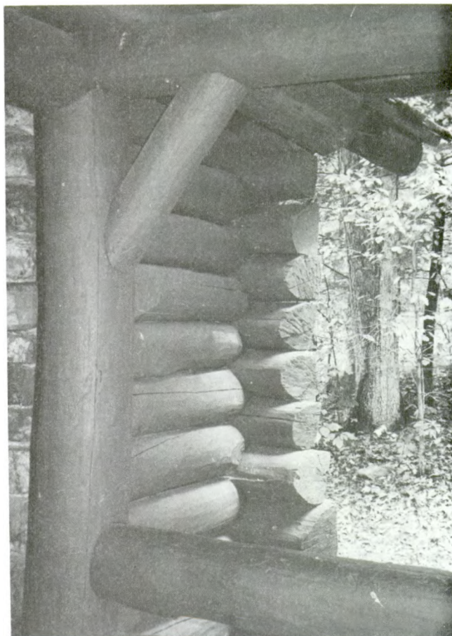
Figure 67--Detail of picnic shelter showing notched log corners and bolted braces, Longdale Recreation Area, George Washington National Forest, VA. (Photo by Kim Lakin, 1982)
