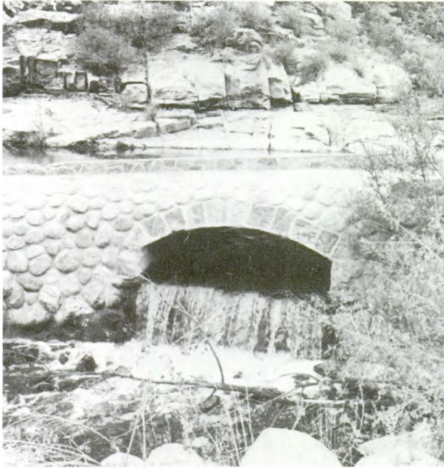
Figure 123--Stone bridge and culvert, Sabino Canyon Recreation Area, Coronado National Forest, AZ. (Photo by Kim Lakin, 1982)
