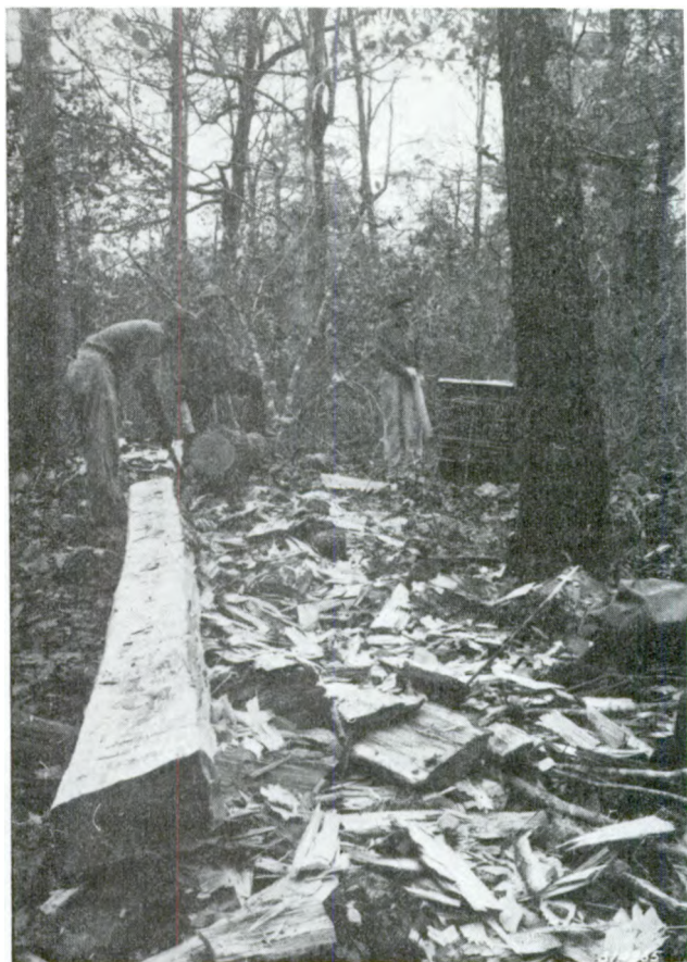
Figure 14--CCC enrollees cutting out shakes for Collier Spring Shelter, Ouachita National Forest, AR. (National Archives 35-N-314335)
