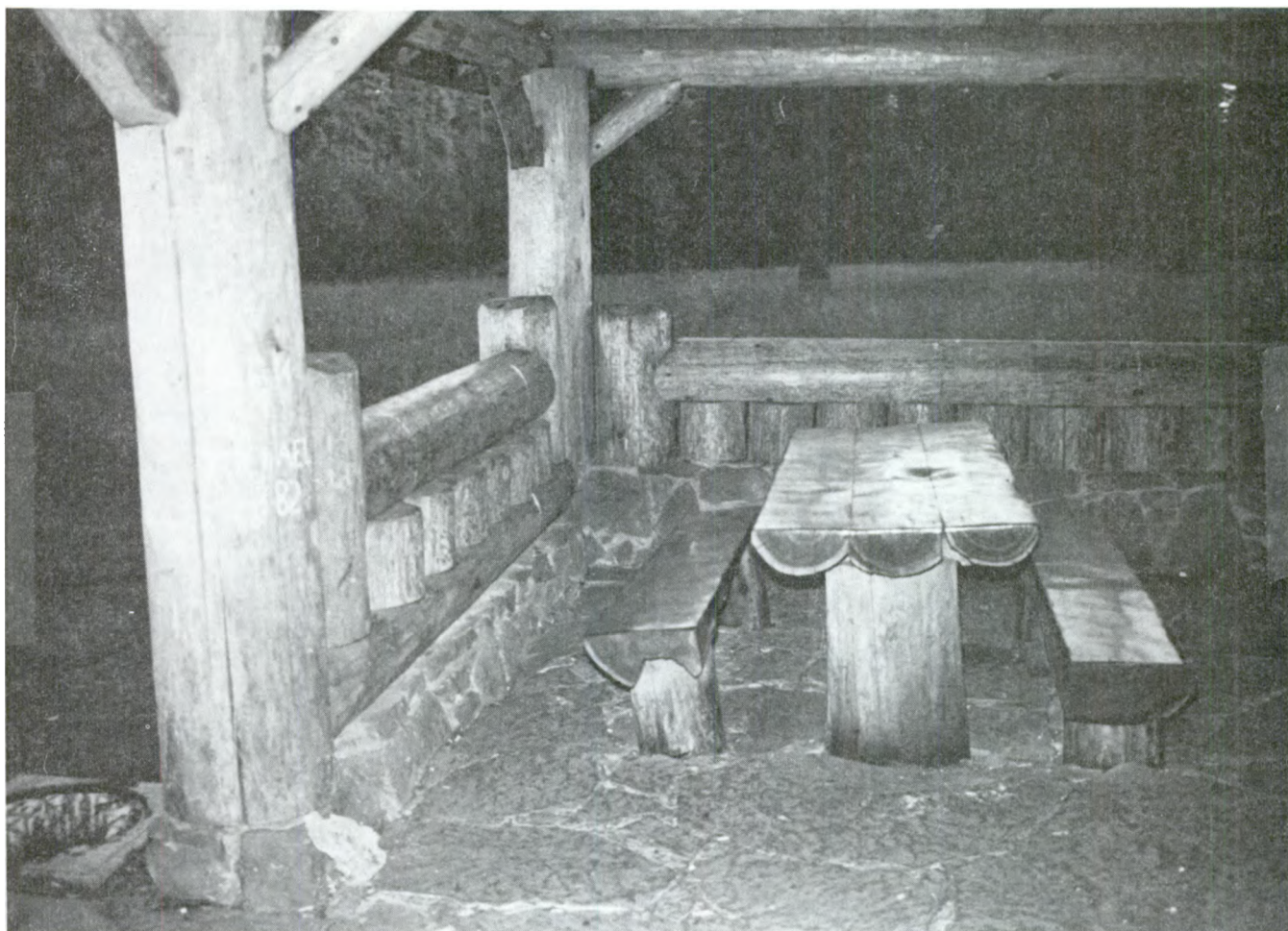
Figure 145--Logs used as railings, window sills, and lintels, Bear Springs Picnic Shelter, Mount Hood National Forest, OR. (Photo by Dennis Egner, 1982)
