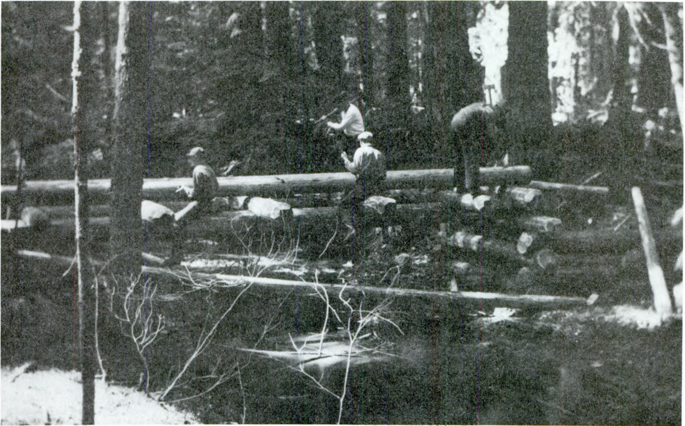
Figure 13--CCC enrollees building log bridge at Dalles Camp, Snoqualmie National Forest, WA, in 1936. (National Archives 35-G-340106)
