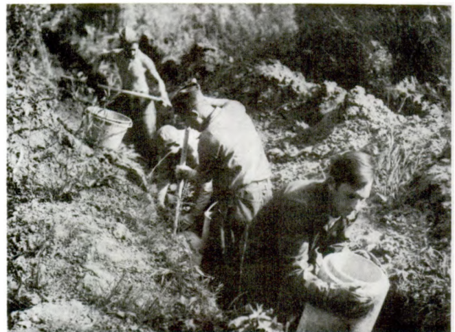
Figure 10—CCC enrollees laying 8-inch pipeline for Pocatello, ID, city water supply. (National Archives 95-G-280106)
