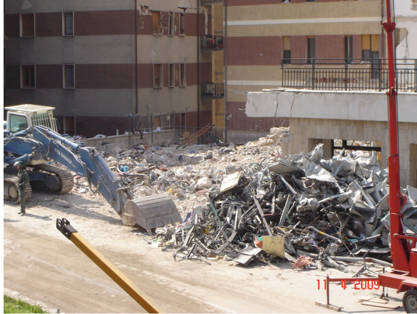
Figure 8 University of L'Aquila, collapsed dorm, 2009. 9
