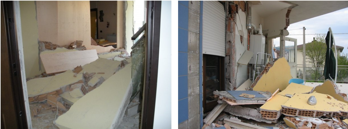
Figure 16 My mom's apartment. Collapsed walls, L'Aquila, 2009.
