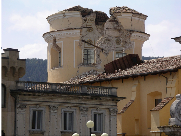
Figure 6 Damage to the roof of a church in the main square, downtown L'Aquila 2009.
