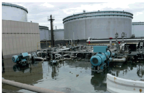
Flooded refinery facilities (Due to a typhoon in October 2019)
