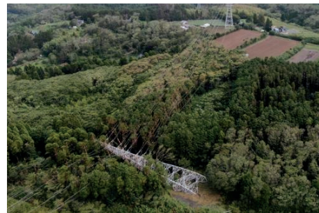
Collapsed power transmission tower in Kimitsu City, Chiba Prefecture (Due to a typhoon in September 2019)
