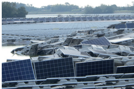
Damaged floating solar power plant in Ichihara City, Chiba Prefecture (Due to a typhoon in September 2019)
