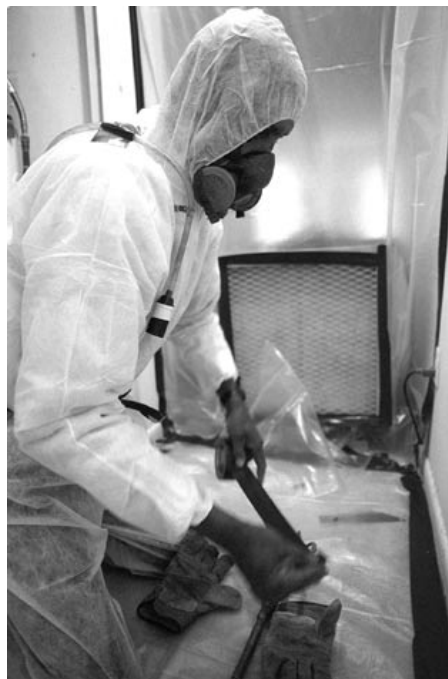
A residential asbestos containment company worker seals a room for asbestos removal in an Atlanta apartment complex. The plastic keeps asbestos particles from settling on the carpet.
