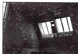
Damage to Erasmus High School
