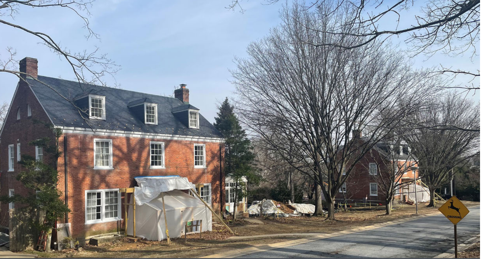
A present day view of 15H and 15I on North Drive. The Bethesda campus residences, originally built in the 1940s, are undergoing renovation.
