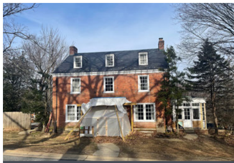
Bldg. 151, one of the "Officer's Quarters" on NIH's main campus, is getting a makeover.
