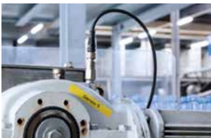
Vibration sensors on the drives detect even smallest vibrations.
