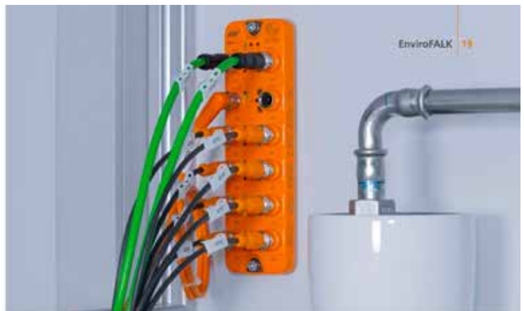
Decentralised IO-Link masters save space in the control cabinet and offer the possibility to connect sensors and actuators. Connection to the plant controller is made via Profinet.
