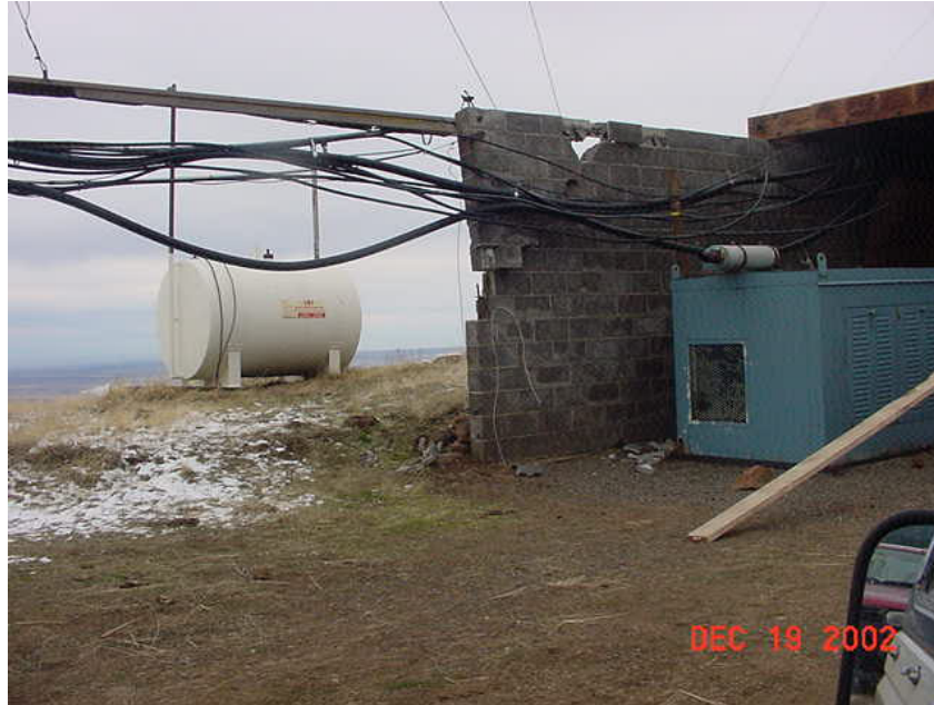
High winds completely tore off a roof over a building and an attached carport at Pike's Peak at 3800 feet.
