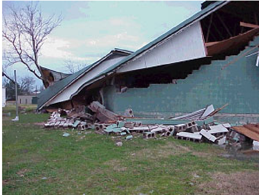
A school bus barn was destroyed by an F1 tornado at Des Arc (Prairie County) on 12/18/2002. No buses were in the barn at the time.
