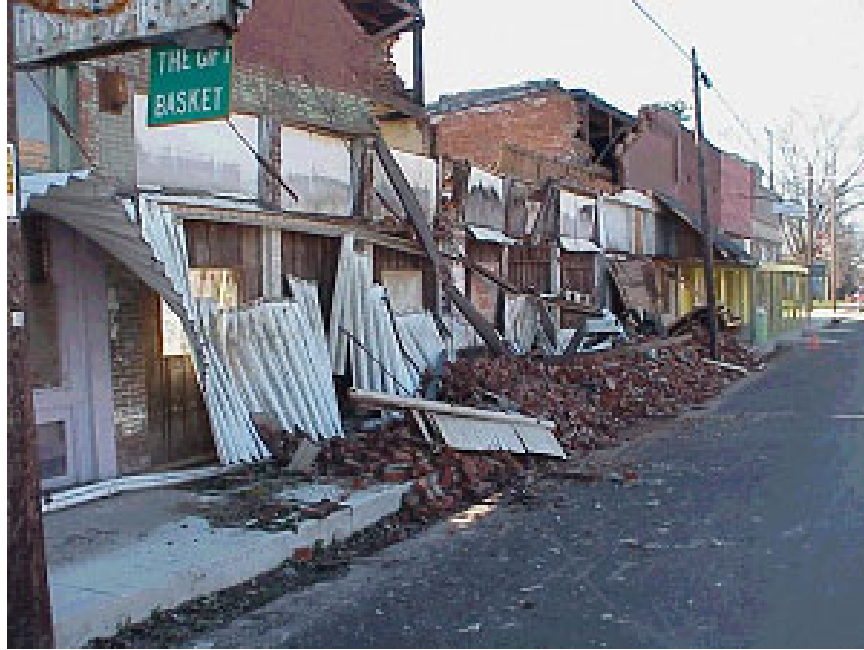
Several building facades collapsed in downtown Cotton Plant (Woodruff County) due to an F1 tornado on 12/18/2002.
