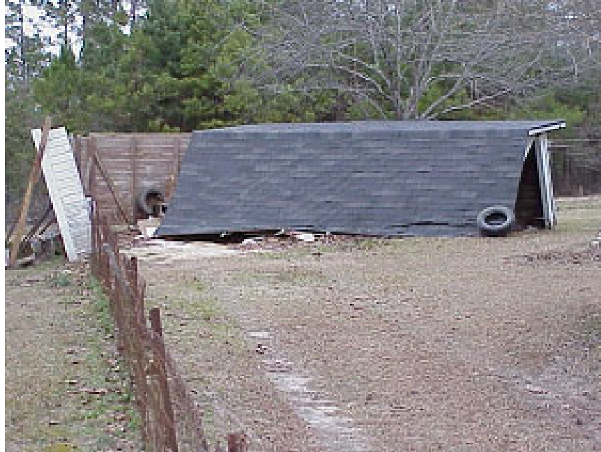
A garage collapsed due to an F1 tornado about 7 miles north of Banks (Bradley County) on 12/18/2002.
