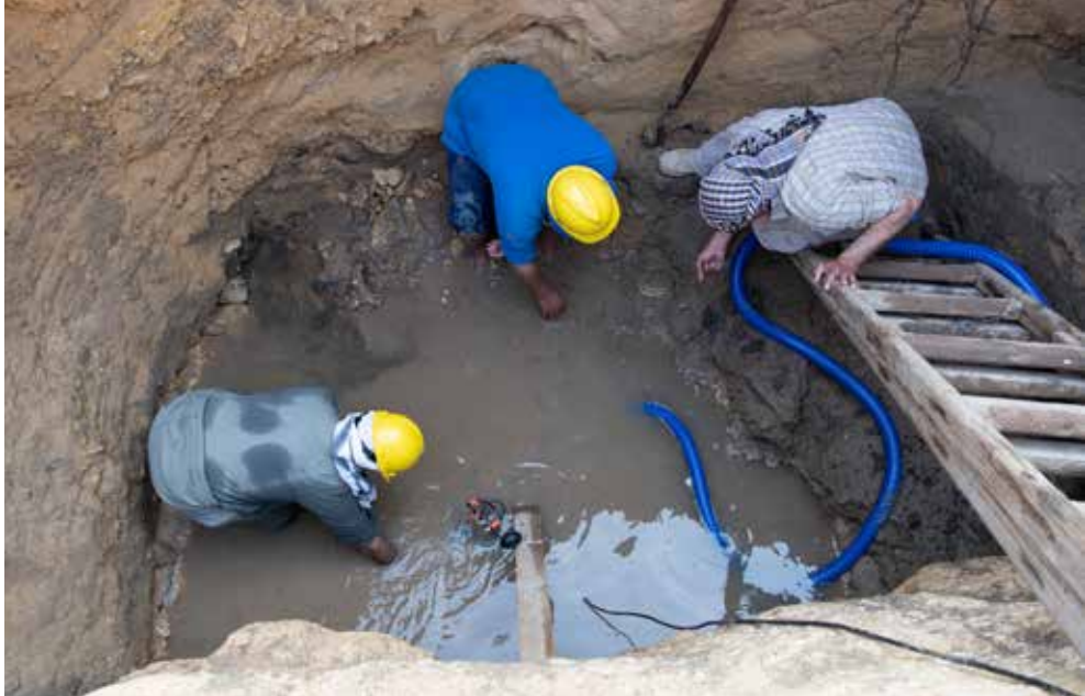
Sayed Salah (on ladder), Ramadan Hussein (left), and Emad Shabaan (center) work with the pump at the bottom of the Dyad Hole. View to the east. Photo by Mark Lehner.
