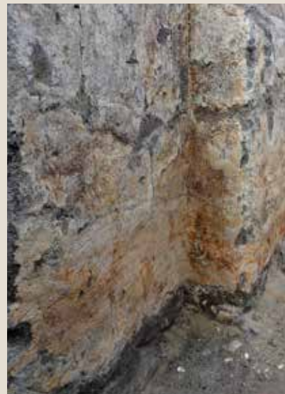
North face of wall, MVT. The rust red paint, although faded (perhaps due to water damage), has survived well on a wall in the MVT. It was applied over white paint, over grayish-brown alluvial mud plaster.
