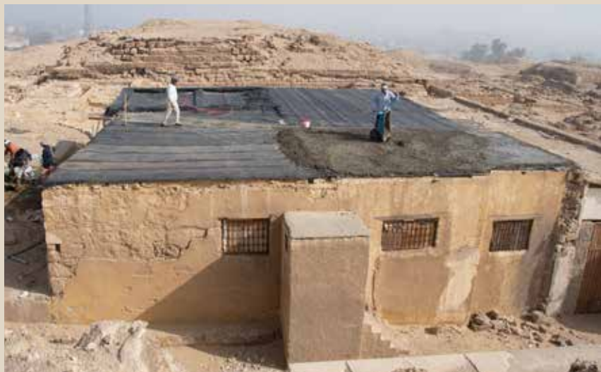
Above middle: Cartons containing archaeological materials spread out to dry. Bottom: Workers spread cement over the new heavy duty plastic that they laid to reinforce the roof. Photos by Mark Lehner.
