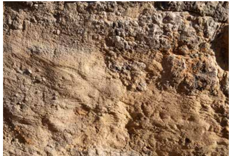
Right: Close-up of the Phase 2 north wall (35,839). Fine sand in the seams of the bricks deposited by streaming water indicates that the temple was left open and abandoned for some time. Photo by Mark Lehner.
