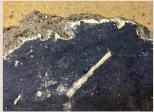
PL133. From KRO, very dark gray plaster applied on white plaster, over grayish-brown mud plaster. The very smooth flat surface shows that it was very carefully made. Many parallel horizontal lines on the surface suggest plastering using a float. The plaster contains many tiny black quartz pebbles, making the surface glitter.
