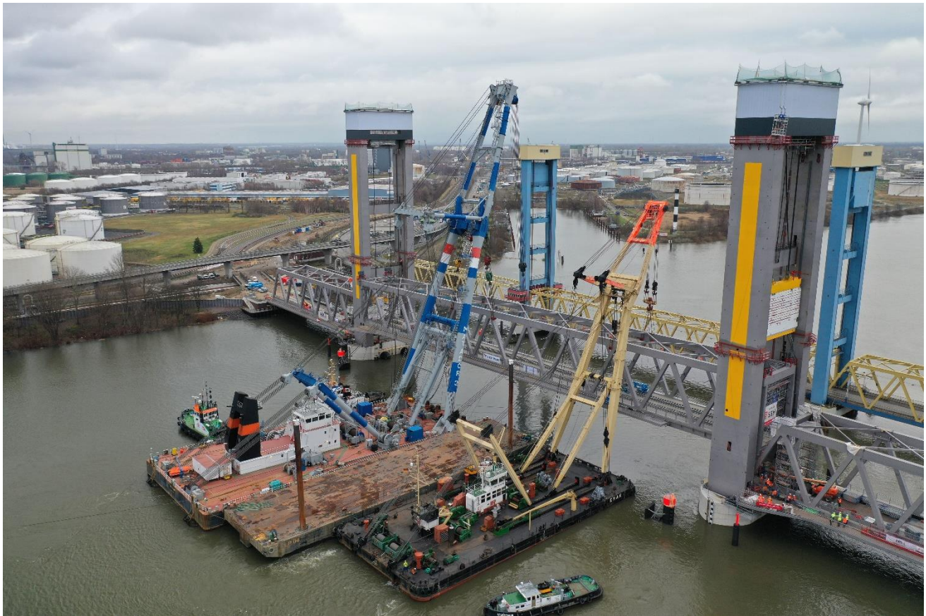
Works on Kattwyk Railway Bridge on the Elbe River (2014-DE-TA-0243-W). Source: Hamburg Port Authority
